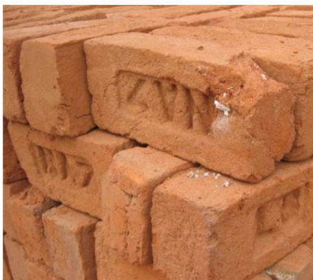
Poor Quality Brick
